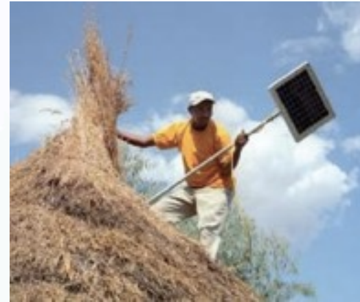
Installations in Ethiopia
