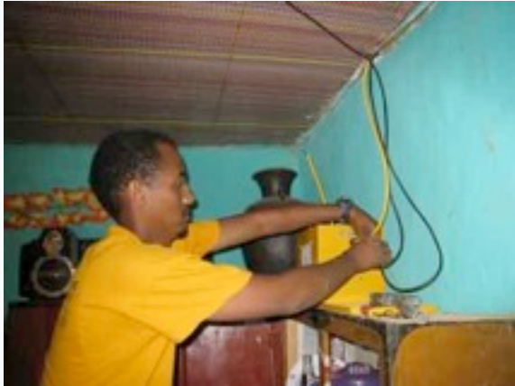
Installations in Ethiopia
