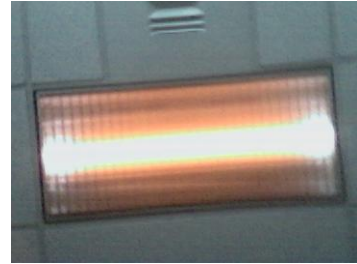
Flourescent lightbulb with grating on it.
